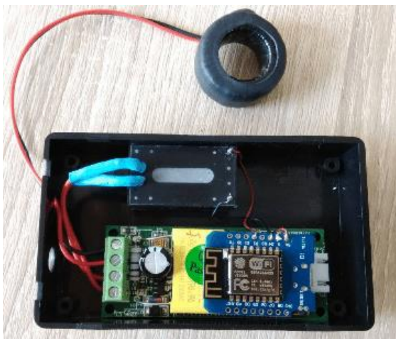
Figure 4. Prototype of an energy monitoring node
